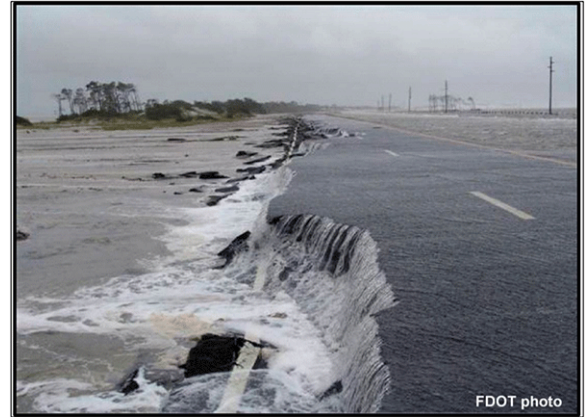
B - Example of the weir-flow damage mechanism as it occurs
