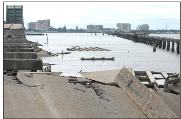
D - Two bridges destroyed by wave loads in Hurricane Katrina
