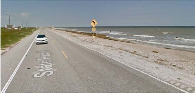
A - Toe Scour causing concrete median barriers to topple along the shoreline adjacent to SH87 near High Island, Texas
