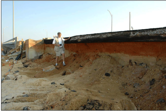
A - Partial embankment damage caused by wave attack
