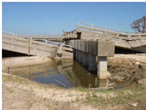
E - Wave scour hole formed by Hurricane Katrina
