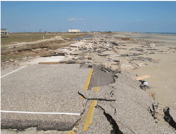
C - Pavement damage due to waves and surge in an extreme event in Brazoria County after Hurricane Ike
