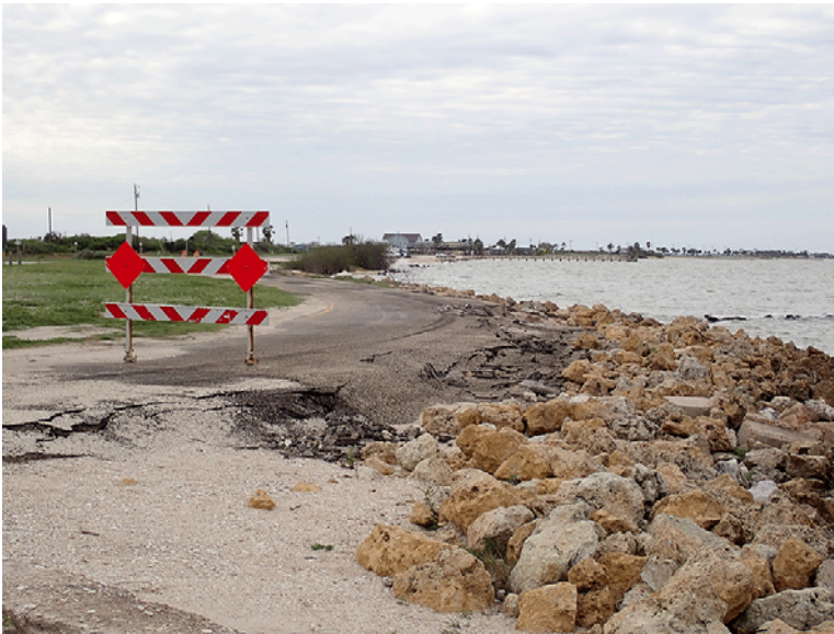
B - Inadequate Armor Layer - A revetment with rocks too small to withstand wave attack along SH316 in Calhoun County, Texas
