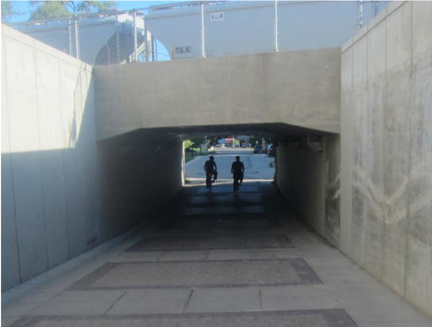
Figure 7-38. Underpasses For Pedestrians And Bicyclists Should Provide Clear Sightlines At The Approach And Through The Underpass.
