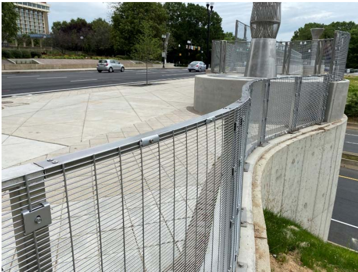
Figure 7-37. A Railing as a Barrier Against a Steep Drop-Off for a Sidewalk Facility at an Overpass.
