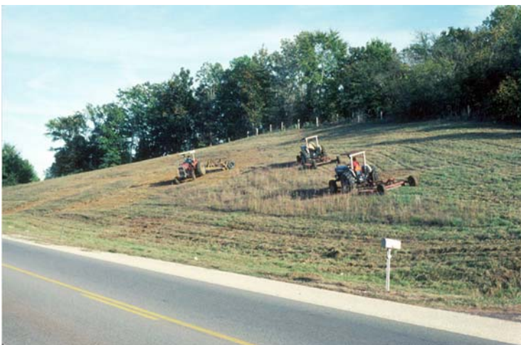
Figure 2-15. Mowing steep slope (rutting and slope failure).
