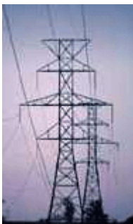
Figure 11-35. Electrical transmission lines.
