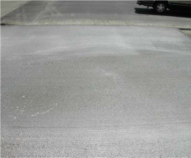
Figure 9-65. Unacceptable – non-uniform application of curing compounds.
