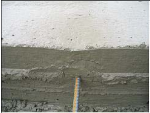
Figure 9-77. Surface drop down due to hand insertion.
