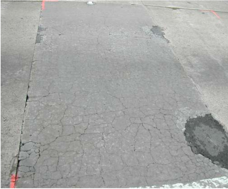
Figure 10-7. Map cracking in FDR slab.
