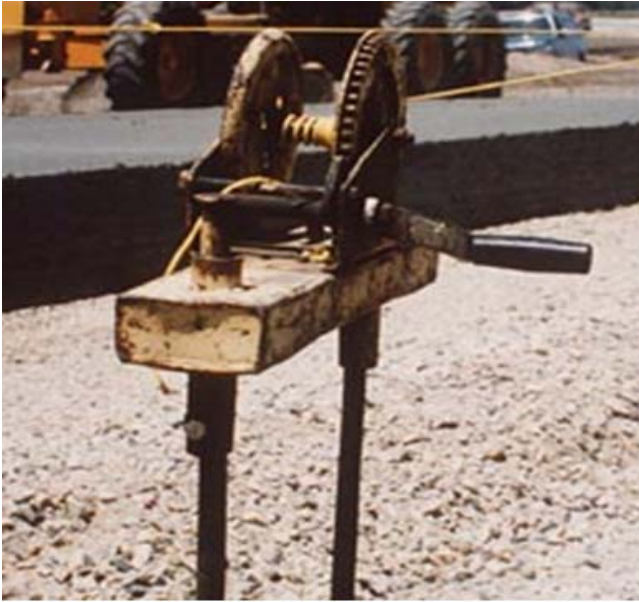
Figure 9-40. Another view of guide wire controls.
