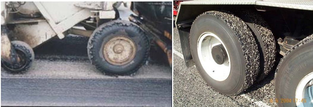
Figure 6-3. Tack coat tracking resulting in no tack coat in the wheel path.
