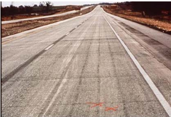
Figure 9-48. Unacceptable – vibrator streaks.
