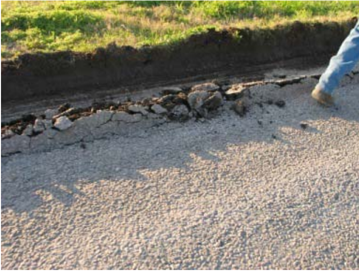
Figure 13-9. Lateral shear failure at the pavement edge (1st photo).
