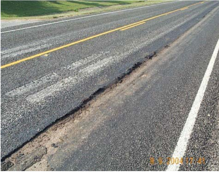
Figure 13-7. Peeling of fresh seal coats (2nd photo).
