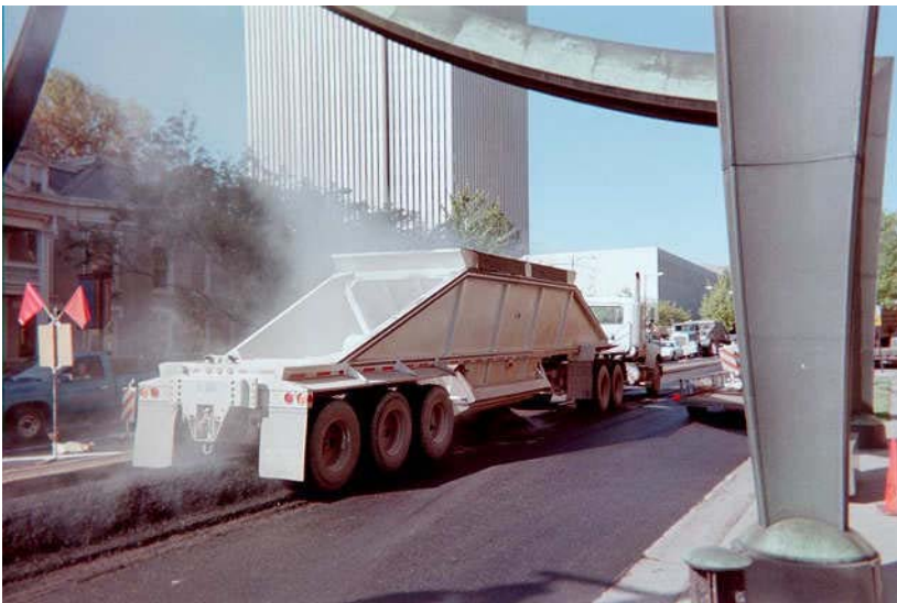
Figure 6-15. Windrow made by emptying a bottom dump truck. © Copyright 2006 University of Washington
