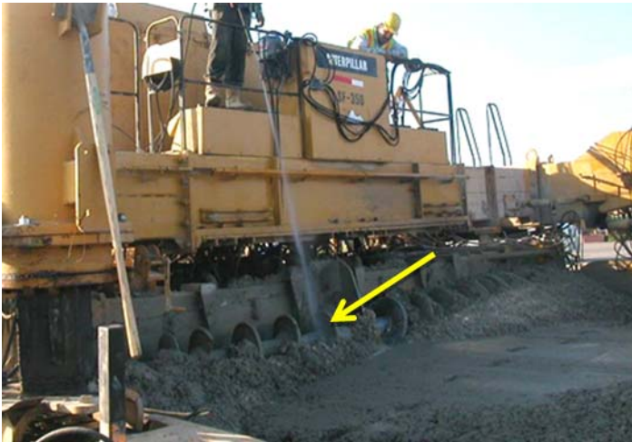
Figure 9-57. Unacceptable - Water being added.
