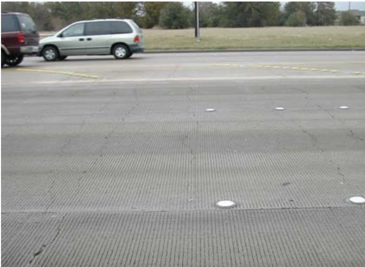
Figure 9-68. Random cracks in CRCP.
