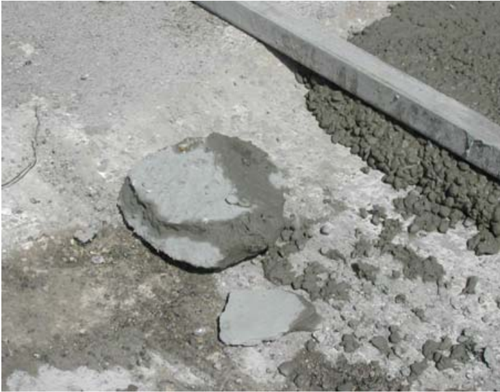
Figure 9-13. Large clumps of concrete.
