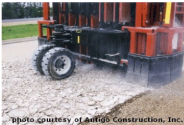
photo courtesy of Antigo Construction, Inc. Figure 7-8. Multi-head Pavement Rubblizer. © Copyright 2006 University of Washington
