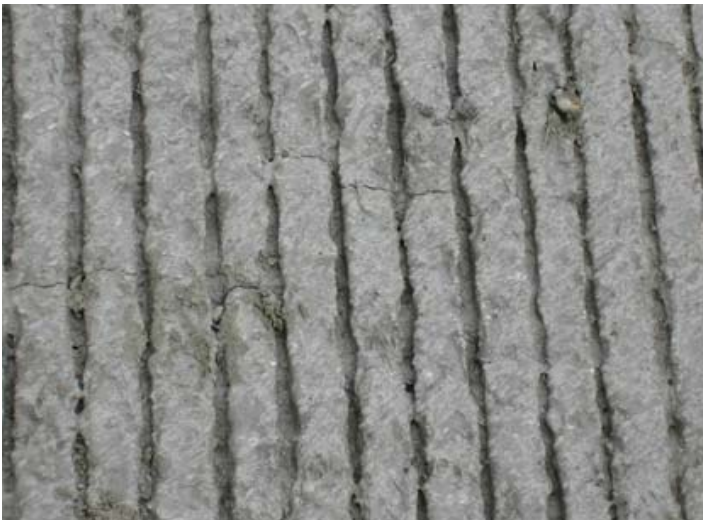
Figure 9-66. Plastic shrinkage cracks.
