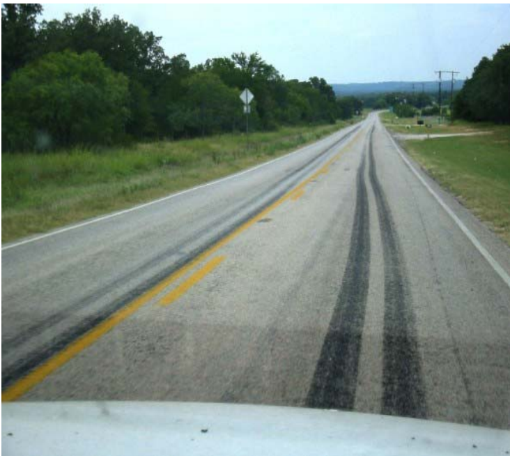
Figure 13-8. Bleeding of seal coats.
