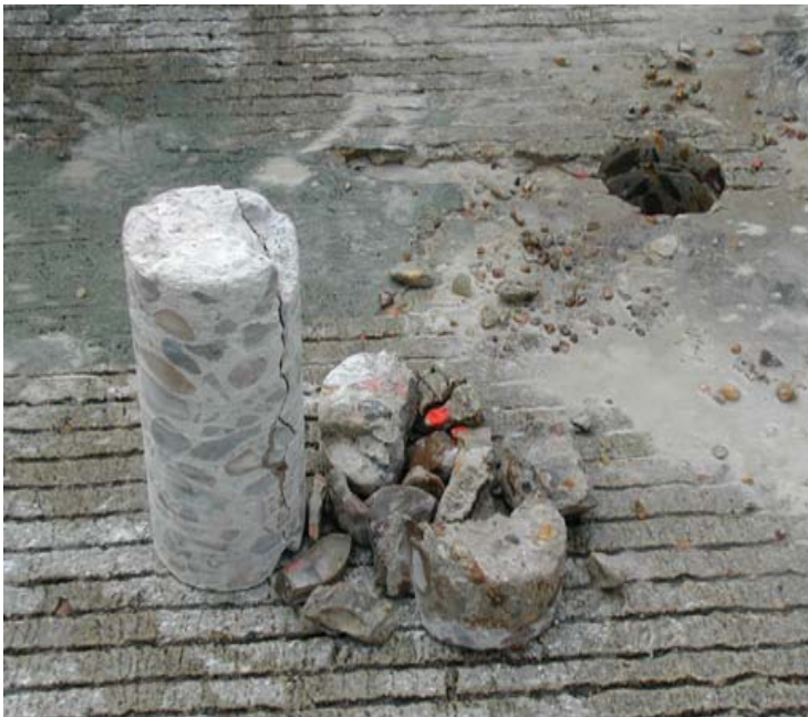
Figure 10-9. Coring adjacent to the spalled repaired area.
