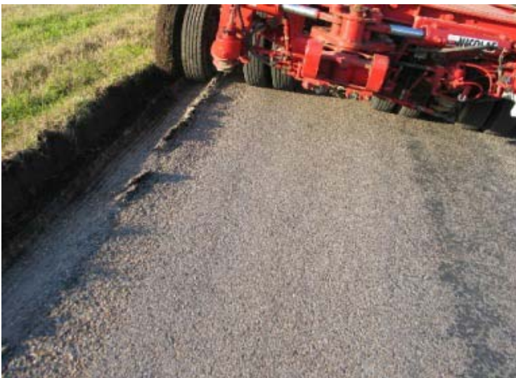
Figure 13-10. Lateral shear failure at the pavement edge (2nd photo).
