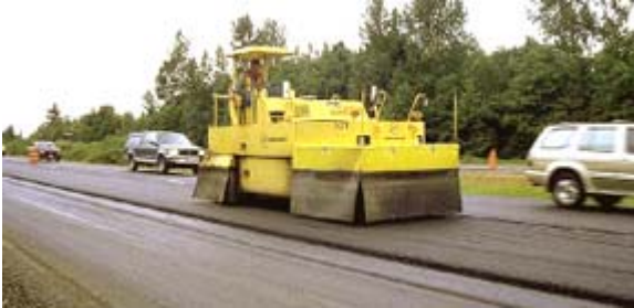
Figure 6-59. Pneumatic Tire Roller (notice rubber skirt insulation around tire area as well as tire marks left in the new mat in front of the roller).
