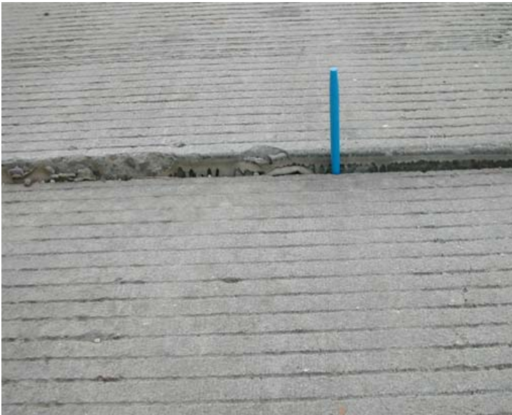
Figure 10-17. Severe faulting at the transverse joint.
