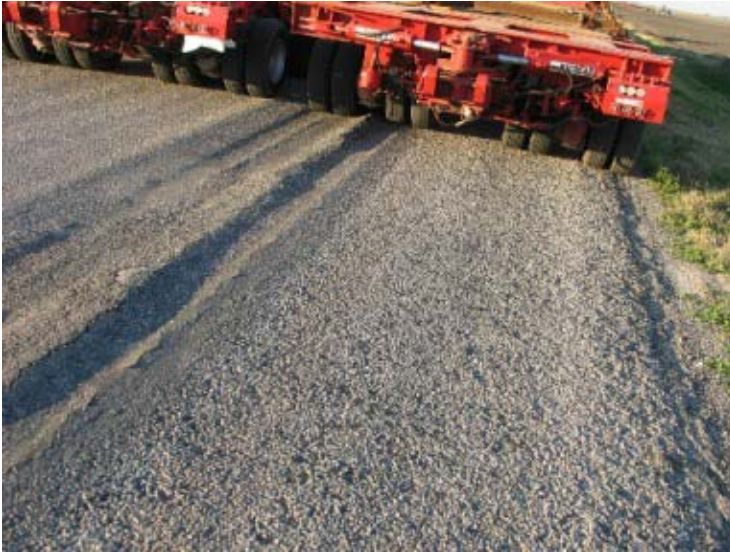
Figure 13-5. Rutting or cracking due to overload of the pavement structure. Recent rainfall or poor drainage conditions resulting in weak or wet subgrade or base materials are often associated with structural damage of this type.
