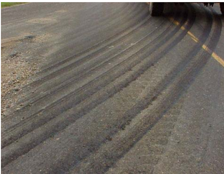
Figure 13-4. Shearing of the pavement surface during turning movements.
