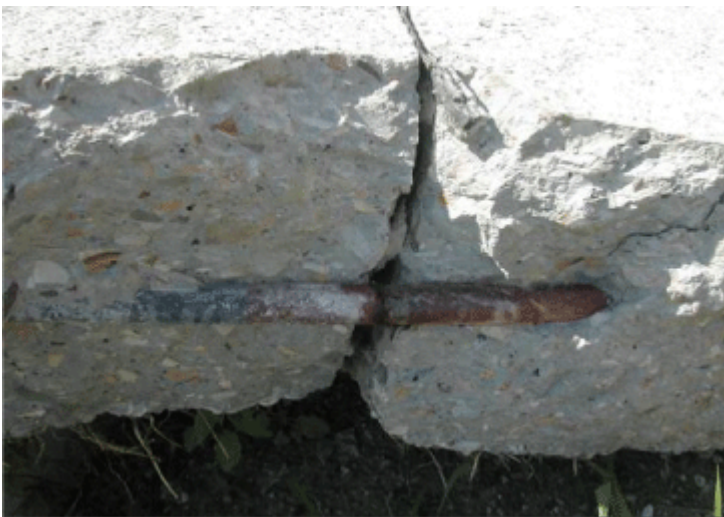
Figure 10-25. Rusted dowel bar.
