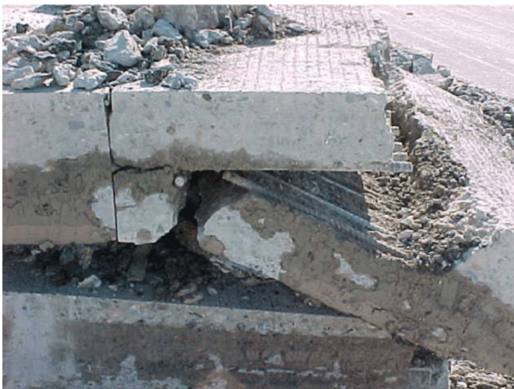
Figure 10-27. Construction joint failure.
