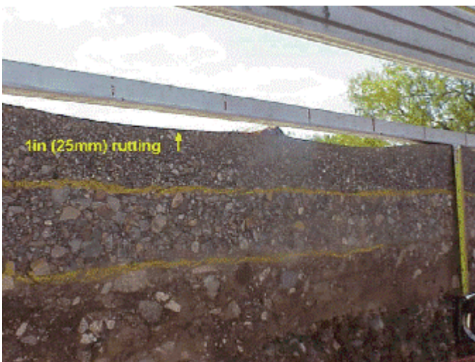
Figure 4-17. Trench sidewalls showing severe rutting.
